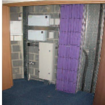
Riser access with purple data cables entering floor void
