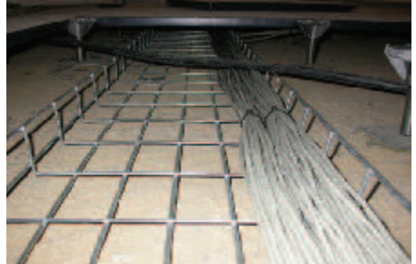
Data cable in tray with power cable running diagonally across the room
